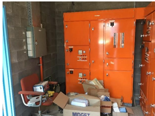
Figure 2-21 Coonabarabran plant MCC (picture 1)
