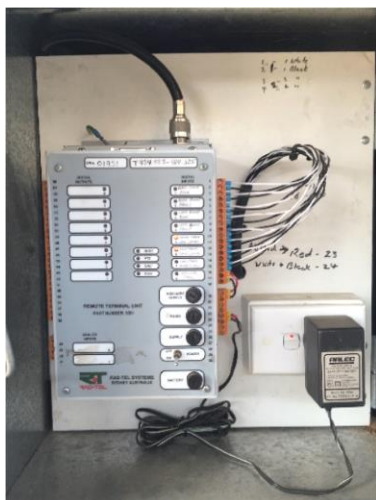
Figure 2-11 Bugaldie RTU internal layout
