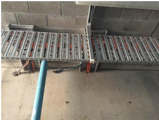
Figure 2-26 Coonabarabran gallery cable tray near filters (picture 2)
