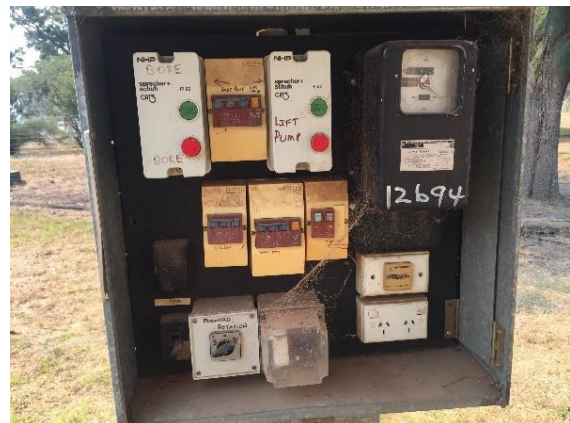
Figure 2-12 Bugaldie control panel
