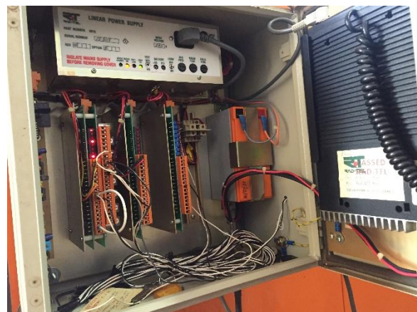
Figure 2-3 Baradine RTU Internal layout
