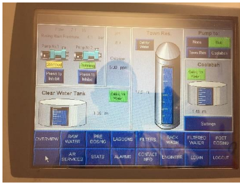
Figure 2-44 Allen Bradley HMI
