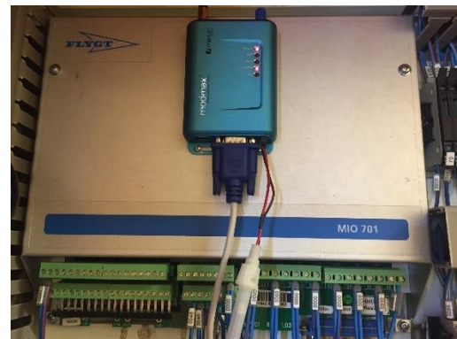
Figure 2-43 Mendooran FLYGT controller
