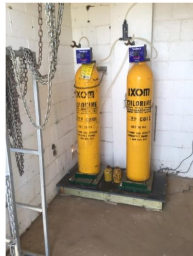
Figure 2-14 Coolah Chlorine bottles and weight cells
