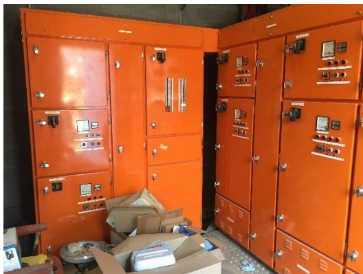
Figure 2-22 Coonabarabran plant MCC (picture 2)
