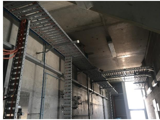
Figure 2-25 Coonabarabran gallery cable tray near filters (picture 1)
