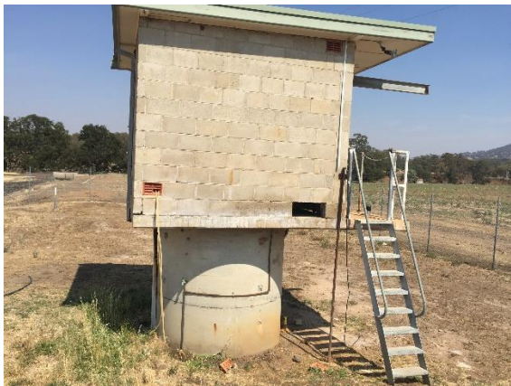
Figure 2-13 Coolah Chlorine dosing room
