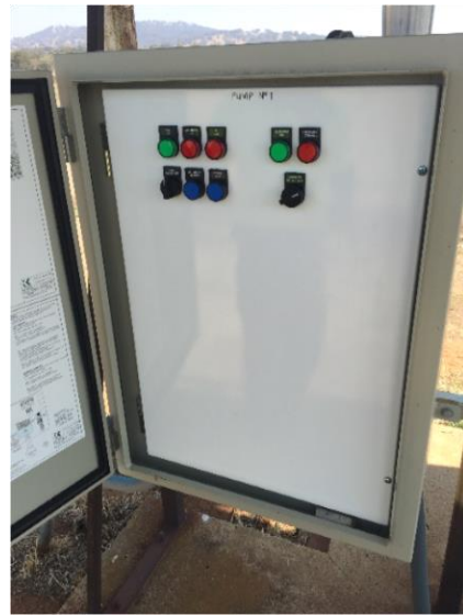
Figure 2-16 Coolah bore pump 2 control panel
