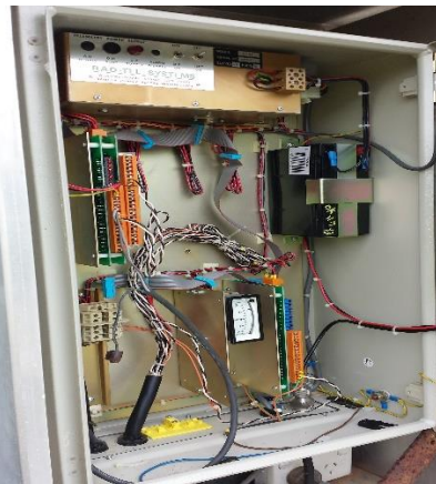
Figure 2-7 Binaway RTU internal layout
