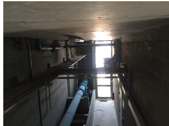
Figure 2-27 Coonabarabran gallery cable tray near filters (picture 3)
