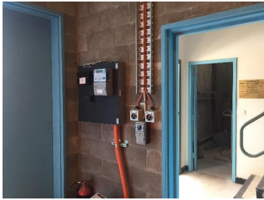
Figure 2-24 Coonabarabran mains power supply to MCC
