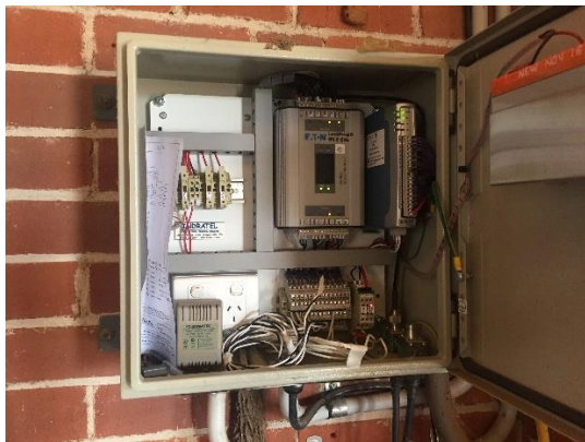
Figure 2-32 Dunedoo RTU panel
