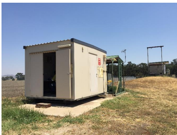
Figure 2-19 Coolah Fluoride dosing room
