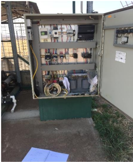
Figure 2-17 Coolah bore pump 1 control panel
