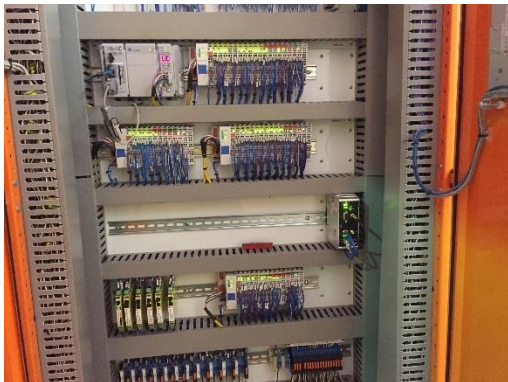
Figure 2-40 Mendooran PLC panel
