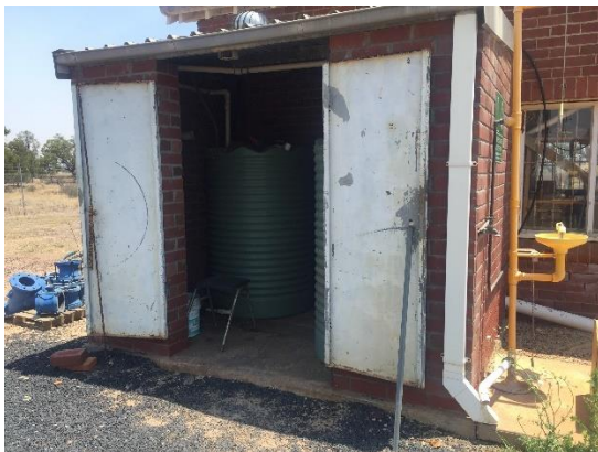
Figure 2-34 Dunedoo Chlorine dosing room
