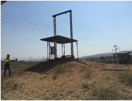
Figure 2-15 Coolah bore pump 2
