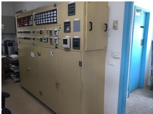
Figure 2-20 Coonabarabran and mimic control panel
