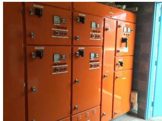
Figure 2-23 Coonabarabran plant MCC (picture 3)
