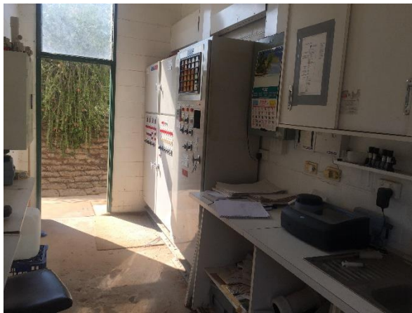
Figure 2-5 Binaway existing MCC
